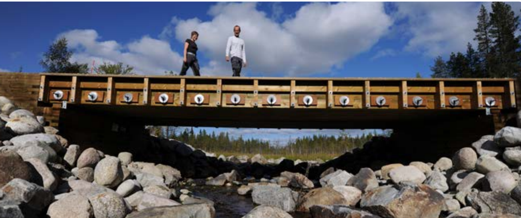
Obstacles for migrating aquatic wildlife are replaced by a wooden bridge that has minimum impact on the aquatic plants and animals. The bridge is made of wood from Holmen's forests. Anna Bylund and Olov Norgren, Rödvattensbäcken, Ångermanland.
